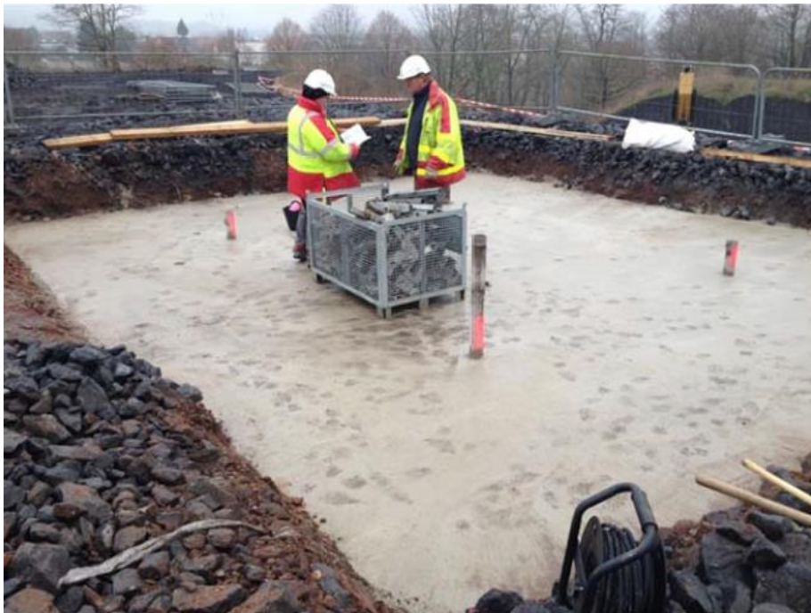
Pictured above is the site of the Obelisk with its piles sunk through a concrete footing! It is finally happening!!
